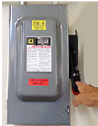
3. Main power OFF .
