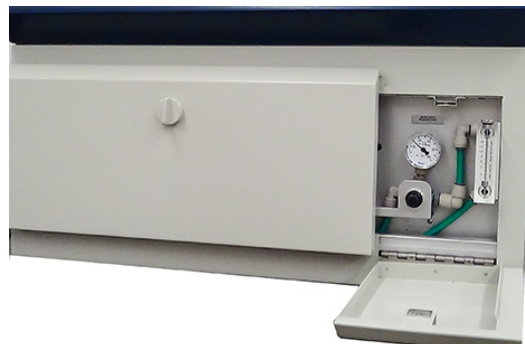
Figure 17.4a: Pressure Gauge, Pressure Regulator, and Flow Meter Location
