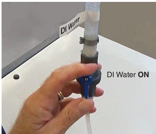
25. Main water supply ON.
