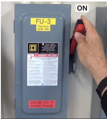
23. Main Power ON.
